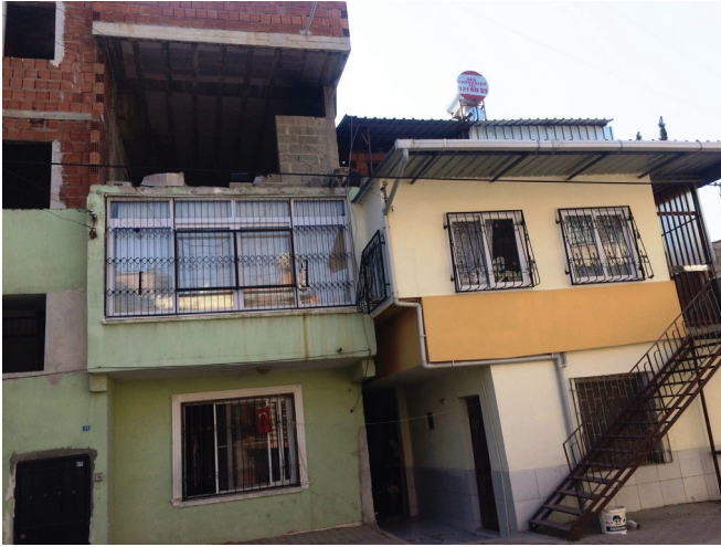
Figure 4-Figure 5. Unsustainable housing constructions in the neighborhood
